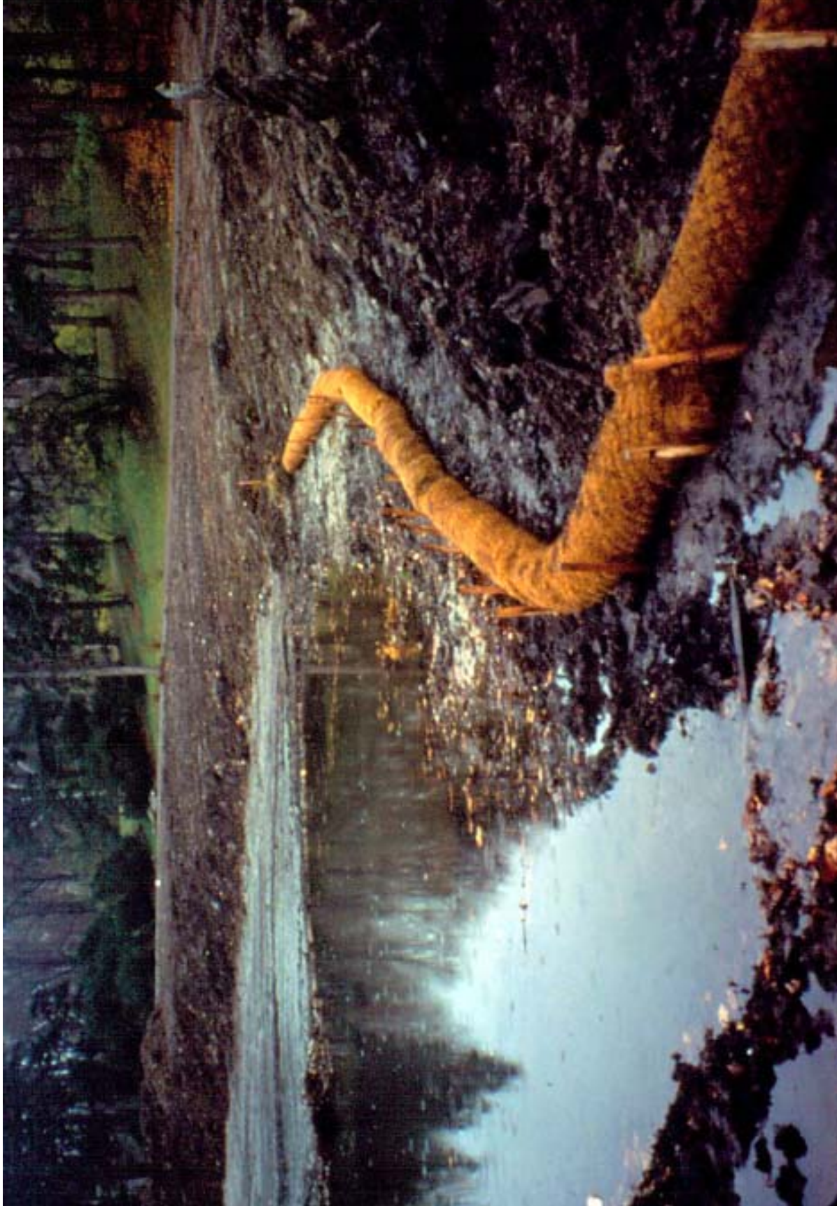
Figure App.C.4 Photograph of bank reshaping and installation of fiber-schine at Trout Pond. LANDSCAPES LA•Planning•HP.
