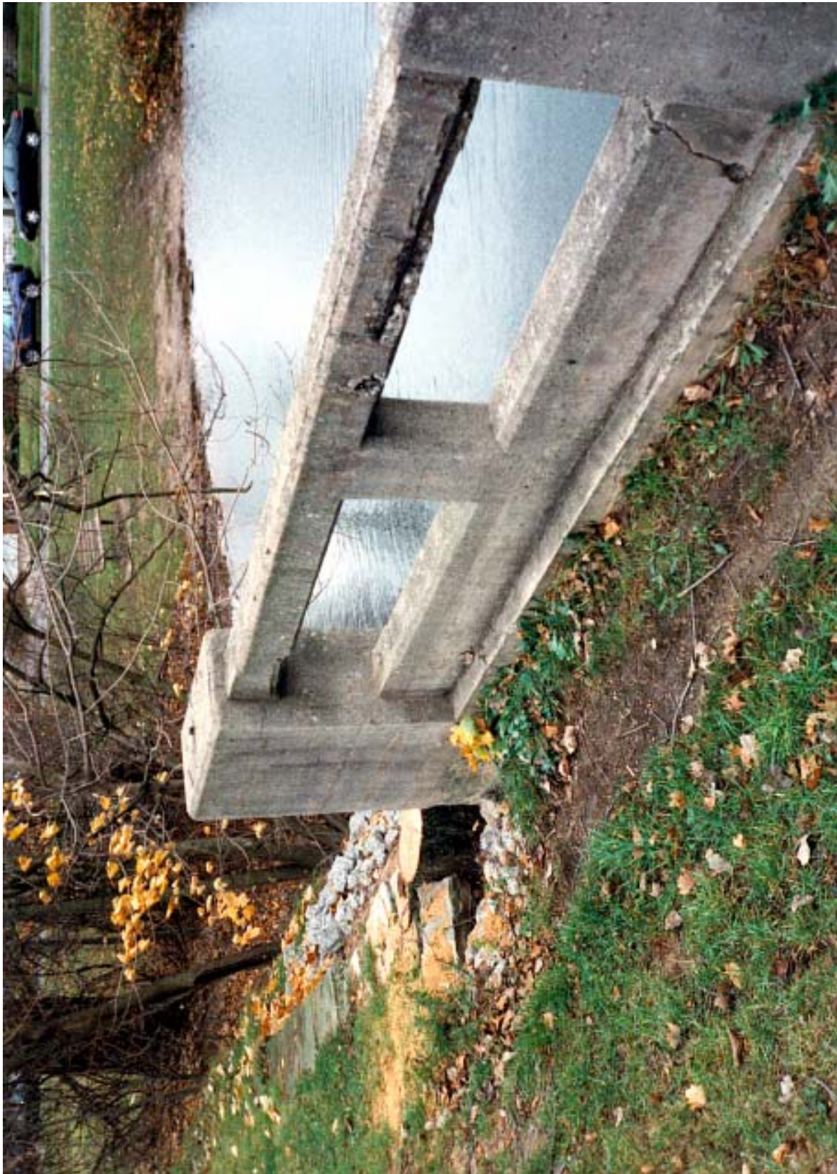
Figure IV.12 Damaged railing and riprap on the bank of the Columbia Avenue vehicular bridge. LANDSCAPES LA•Planning•HP.
