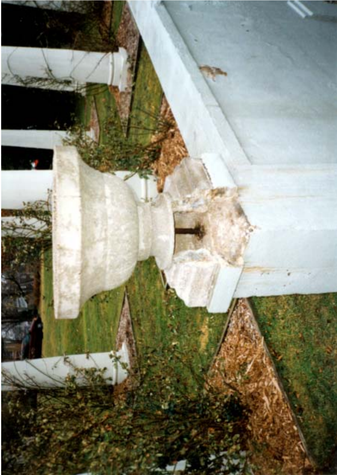
Figure IV.4 Damaged base of urn and wall in the Sunken Garden. LANDSCAPES LA•Planning•HP.
