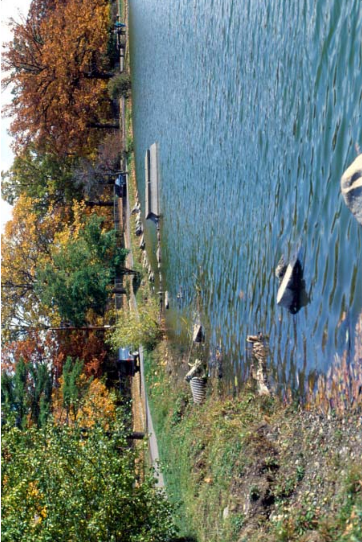
Figure App.C.2 Deteriorated banks of Trout Pond showing eroded edge conditions, 1989. LANDSCAPES LA•Planning•HP.
