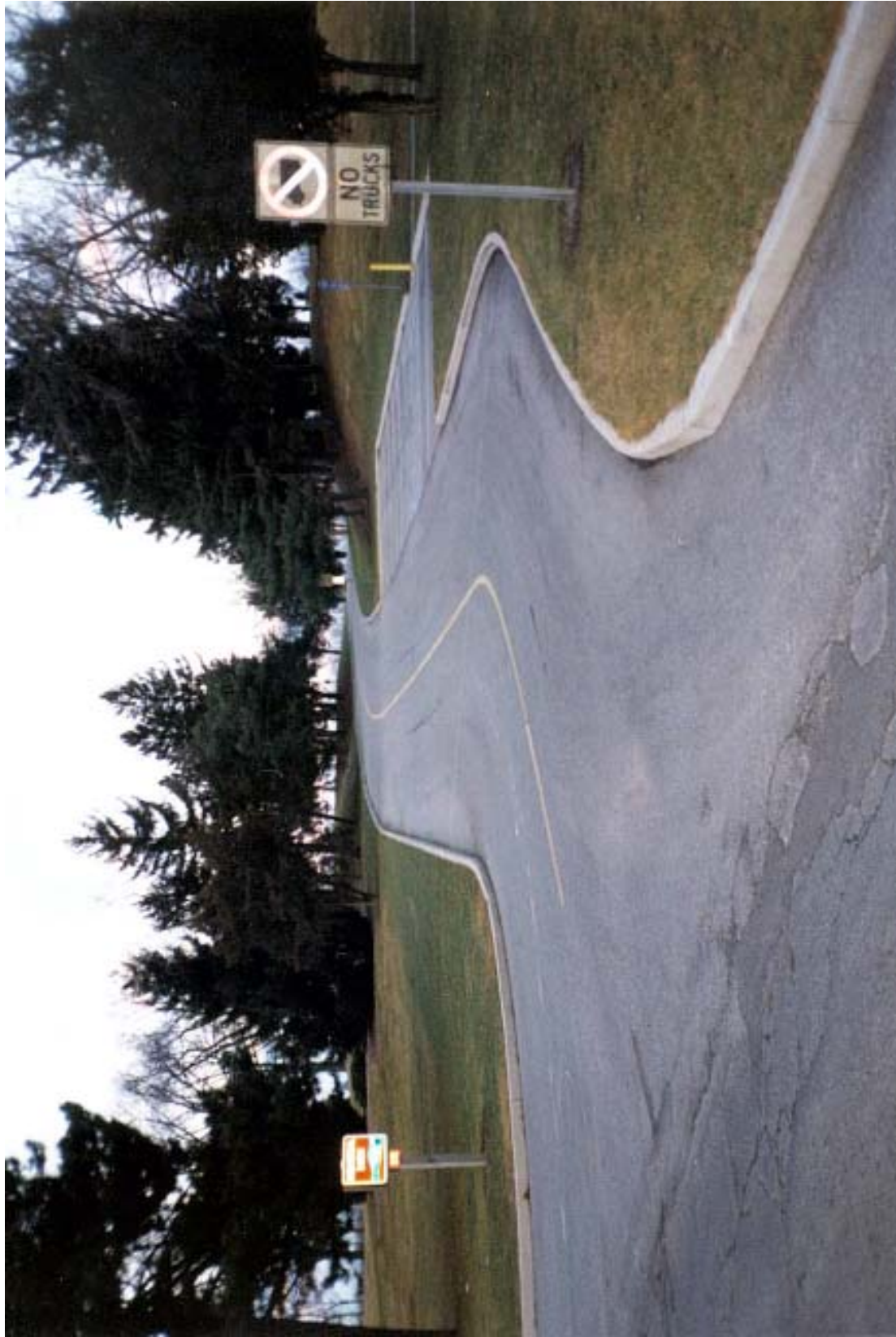
Figure IV.6 The entrance drive has been widened, paved, striped, and curbed, but follows its original alignment. The small parking lot is the first feature you see upon entering the park. The evergreens are remnants of the original c.1928 plantings. LANDSCAPES LA•Planning•HP.
