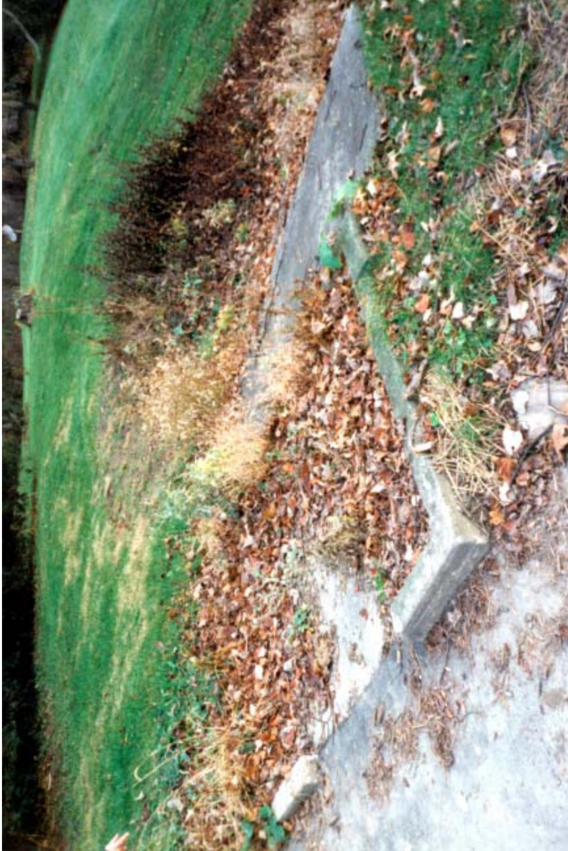
Figure III.17 Remnant foundation of one of the pedestrian entrance arbors near the Greenwood Avenue entrance. LANDSCAPES LA•Planning•HP.
