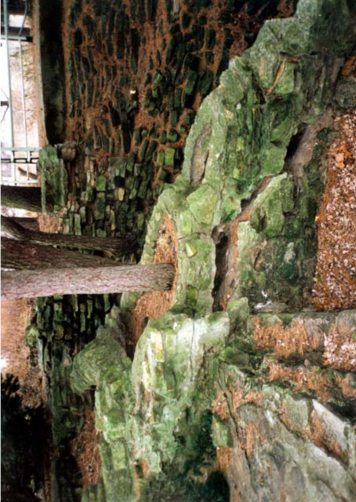
Figure IV.9 Contemporary view of the upper portion of the rockwork of the west waterfall, which is no longer functional. LANDSCAPES LA•Planning•HP.
