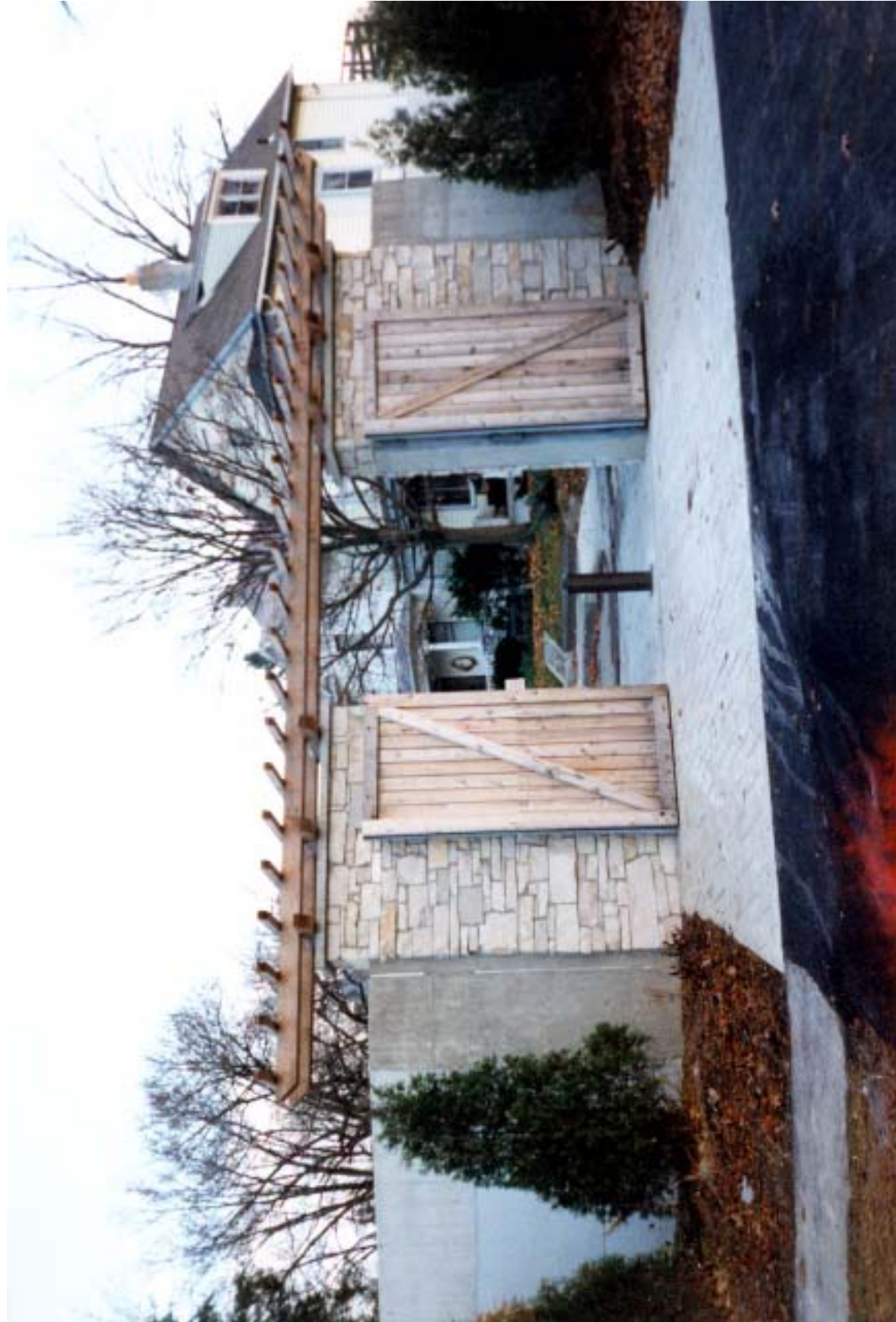
Figure III.16 The recently completed floodwall and grand pedestrian entrance into Swinney Park from Greenwood Avenue. LANDSCAPES LA•Planning•HP.
