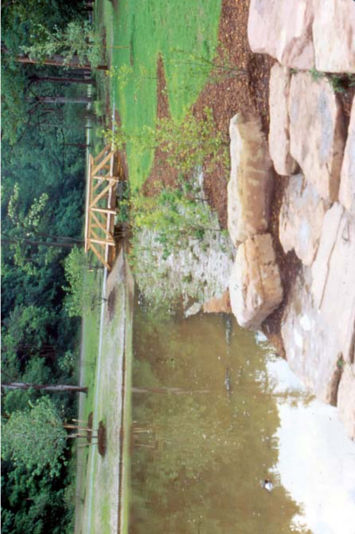
Figure App.C.7 Access area with stone construction shown at intersection with stabilized, planted pond bank. LANDSCAPES LA•Planning•HP.
