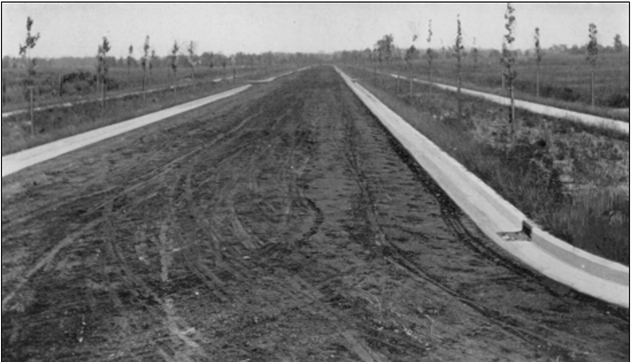
Figure II.7 View looking along Rudisill Boulevard during improvement efforts. Here the standard boulevard scheme devised by the Park Board is evident. The 100-foot right-of-way included a central 40-foot travel lanes edged with concrete curbs. Concrete sidewalks lined either side of the roadway. Park strips lined each side of the sidewalk and were planted with double staggered rows of Oriental planetrees underplanted with mown turf. Initially, the boulevard was unpaved. Courtesy Fort Wayne Parks and Recreation. (R-FTW-RUD-PD-Brd-Rpt-Road-1914.jpg)
